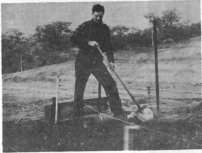
WAYNE LONG FINISHES HOLE FOR SEPTIC TANK AT HIS HOME SITE ON SO. GRADE ROAD. BULLDOZING BY FRED RUSHING.
